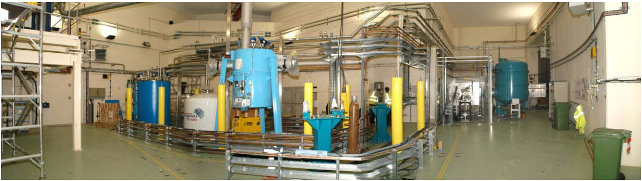
Figure 5: 4 K and 2 K vessels and cold box in place.
