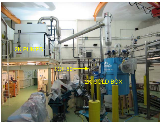
Figure 7: Commissioning of the ERLP Cryogenics.
